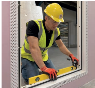
Adjust the position of the frame using the jacking screws to ensure it is aligned vertically and horizontally within the structural opening.
