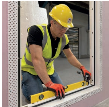
Adjust the position of the frame using the jacking screws to ensure it is aligned vertically and horizontally within the structural opening.
