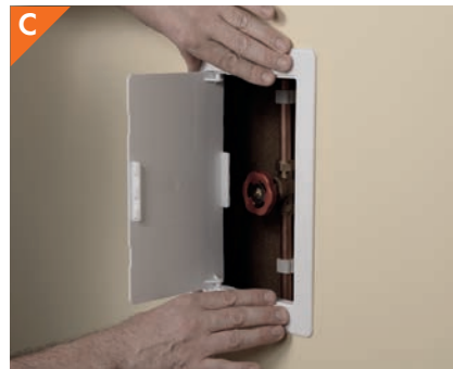
It is held in position to bond the plastic access panel into place
