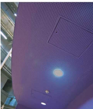
Profab access panel into Rigitone ceiling at the Curve Performing Arts Centre Leicester
